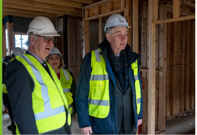
Cliff Barclay, Baptcare Affordable Housing with former Victorian Housing Minister Richard Wynne, and local member Natalie Suleyman MP visiting Sunshine PassivHaus building site in June.
